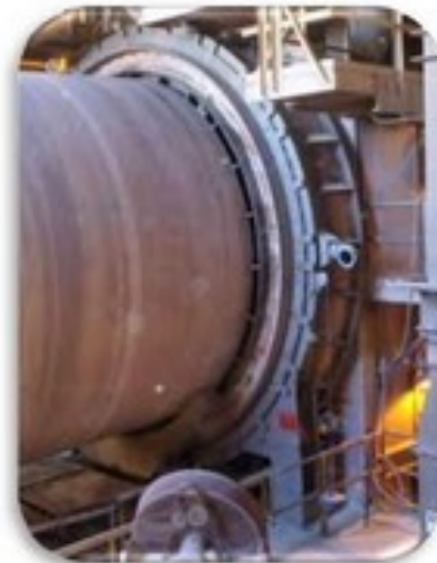
Kiln Inlet Seal
