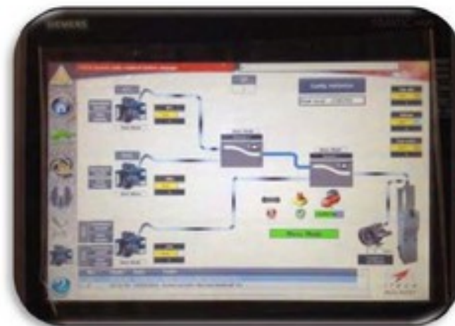
Touch panel for control
