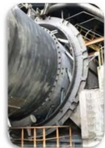
Kiln Outlet Seal
